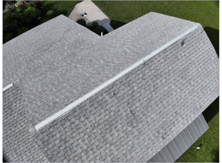
Photo 4: Ridge vent run and rear slope, dark marks near ridge end
