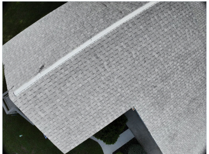
Photo 12: Ridge vent and rear slope, dark area at ridge end
