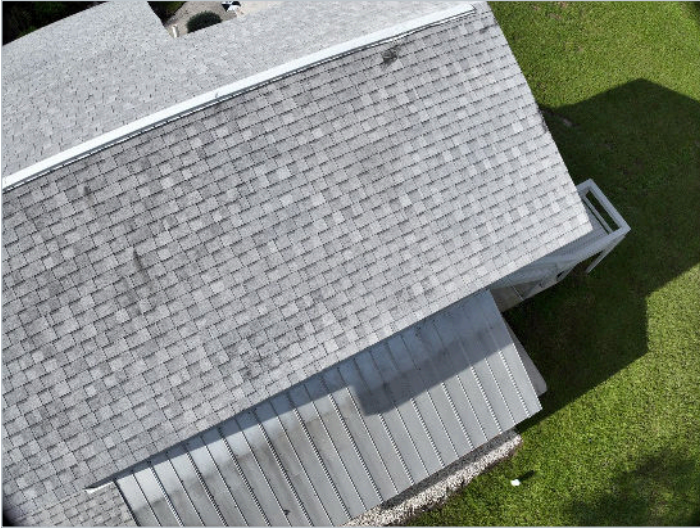
Photo 3: Rear slope and lean-to metal roof, dark streaking at ridge
